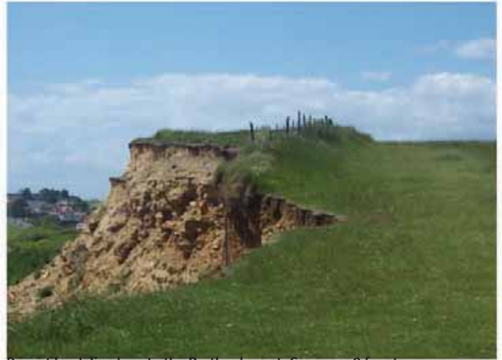
Recent landslip close to the Portland coast. See page 9 for story. Photograph courtesy of Weymouth & Portland Borough Council
